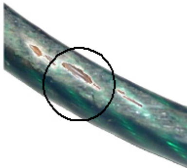
Figure 5. Damaged plastic coated wire rope.
